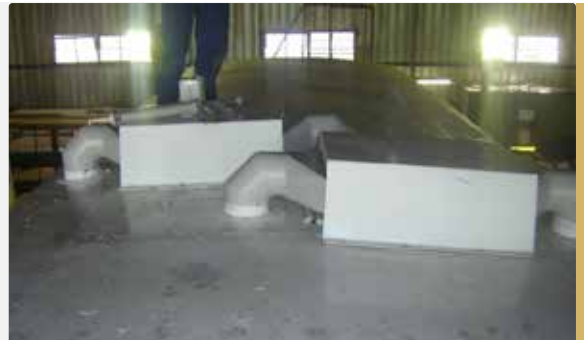
Fan and air ducting system on Harmony bus.
