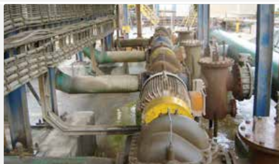
Kusasaletu energy-saving project
