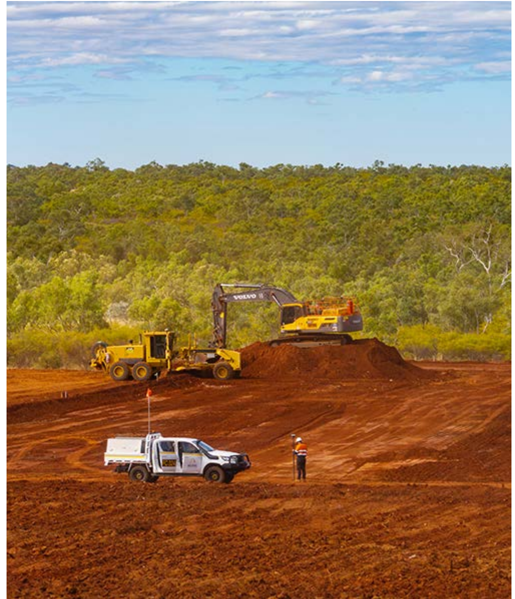
■ The high availability of solar energy/resources has been integrated into Eva Copper design
