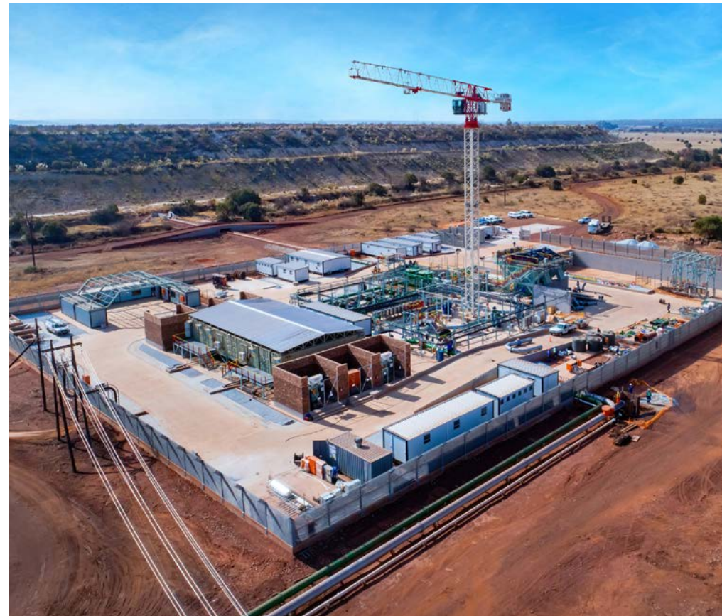
■ Mine Waste Solutions 4 and 5 pump station
