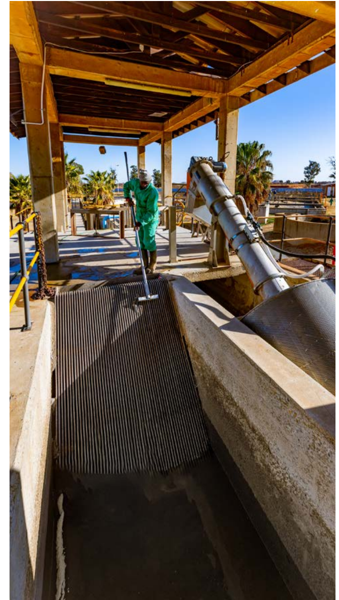
■ Water management at Oberholzer Wastewater Treatment Plant
