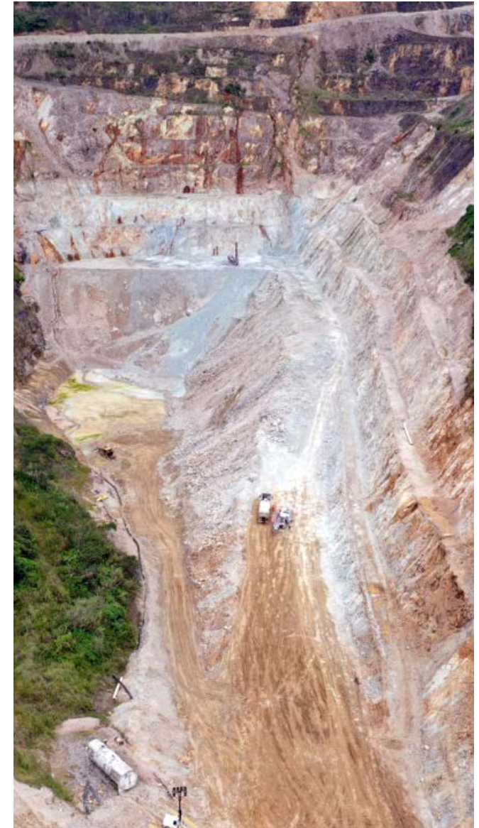
■ Construction activities to convert Hidden Valley's Hamata open pit to TSF 2 commenced in FY24
