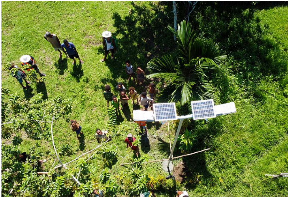
■ Solar streetlight at Mundala, Wafi-Golpu
